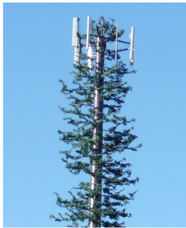
Cell Phone Antenna (disguised)
